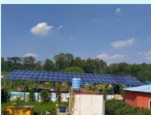
Solar power plant at Wai FSTP
