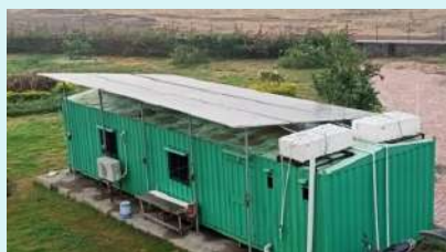
Solar power plant at Sinnar FSTP
