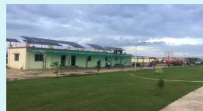
Solar power plant at Bhubaneshwar FSTP
